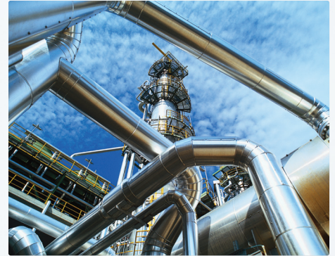
Chemical, Oil and Gas
